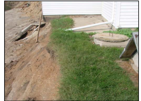
Washed away SSTS in eroded stream bank
